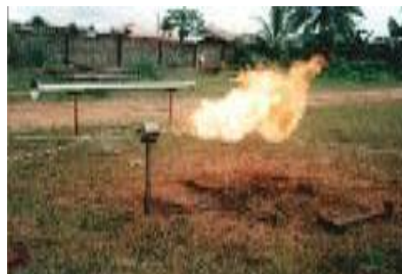
Pilot burner ignited by Elyxxon flare ignition torch
